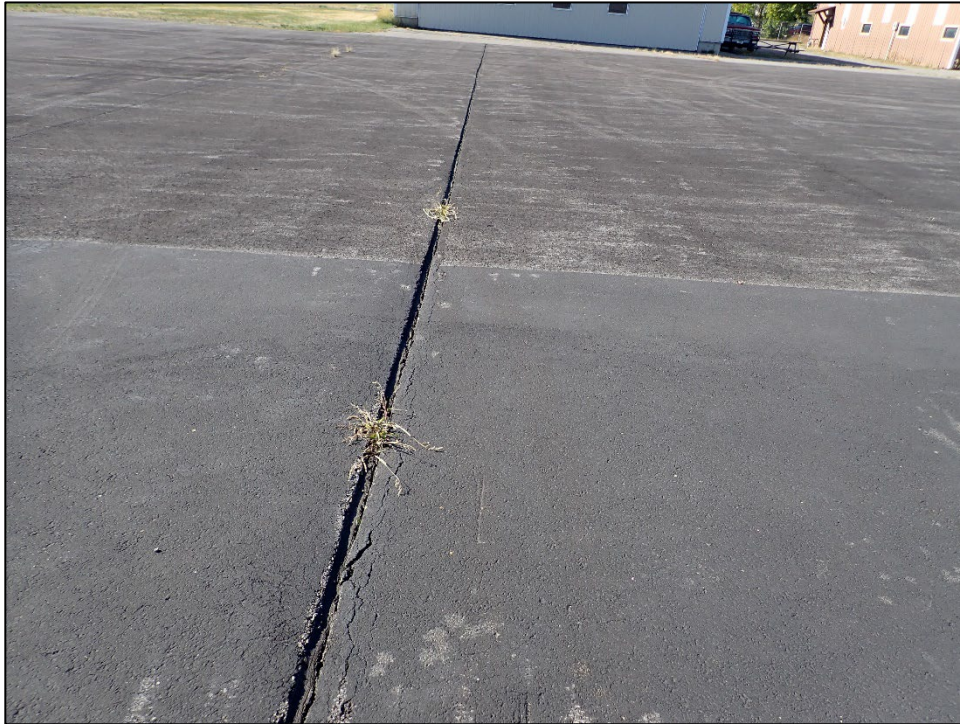
AP-11-07: L&T Cracking
