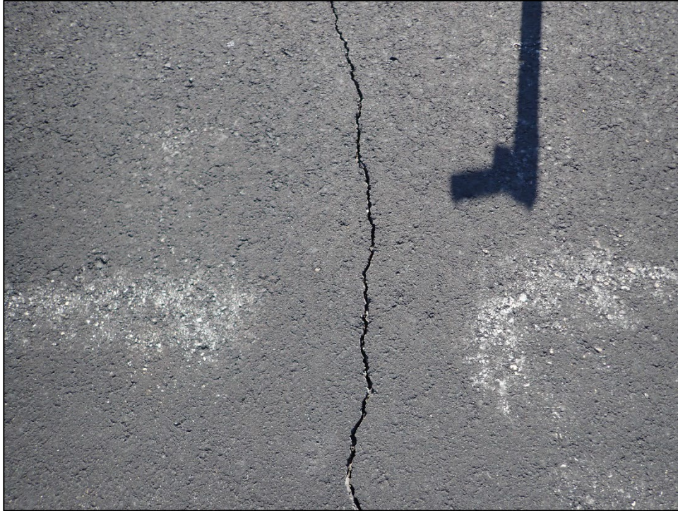
RW10-01-20: L&T Cracking
